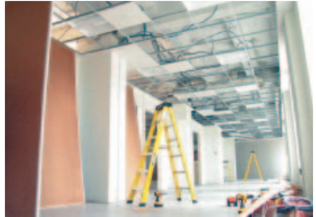
With FlexHead they only had to do one drain-down, saving time, money and water. Saving water is consistent with green objectives and the project achieved LEED Gold Status.
