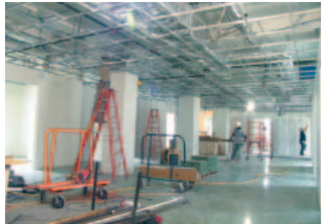
FlexHeads were installed, tested and out of the way so that the other trades could work without worrying about sprinkler piping or contractors getting in the way.
