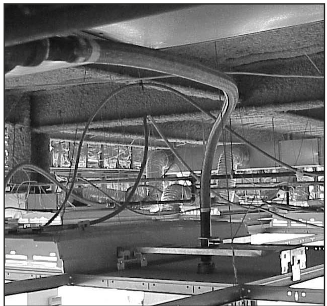
High-quality flexible systems deliver substantial net gains in cost and time over hard pipe armovers, whether measured by per-head or by hourly productivity criteria.
